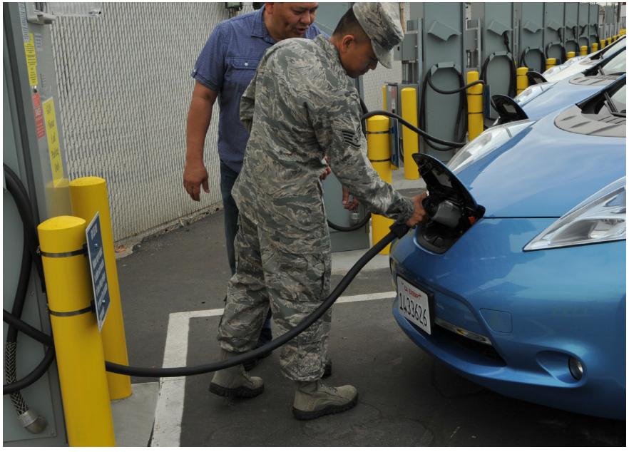
Princeton Power Systems' EV Charging Technology being utilized at the Los Angeles Air Force Base.
